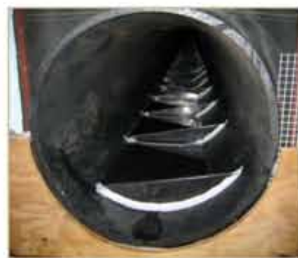
Baffled Culvert (UWRL)
