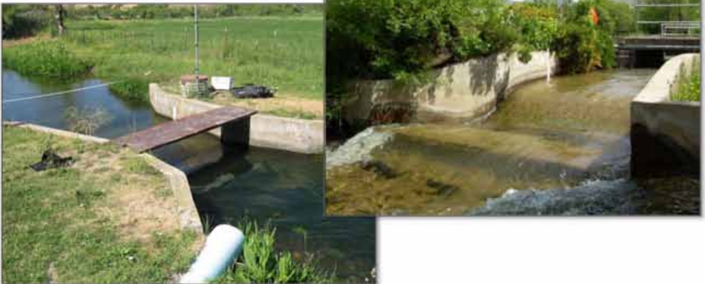
Examples of Flow Measurement Devices Tested in Utah
