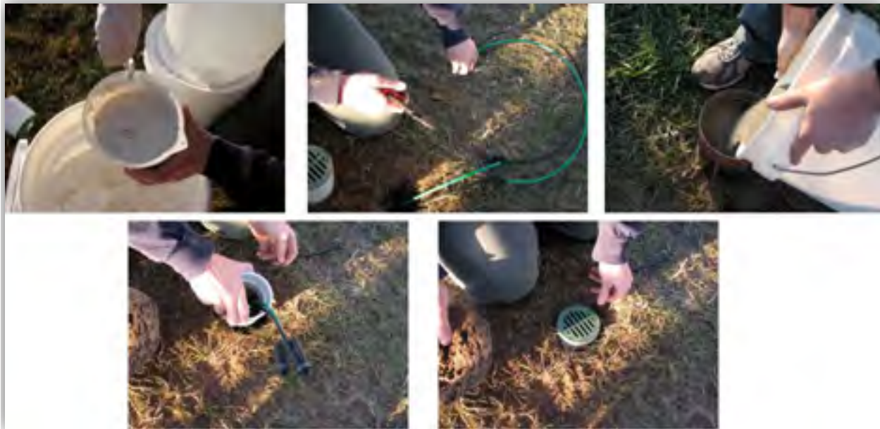
Installation of lysimeters using silica and bentonite. Access tubes extend to surface and are covered with a grate
