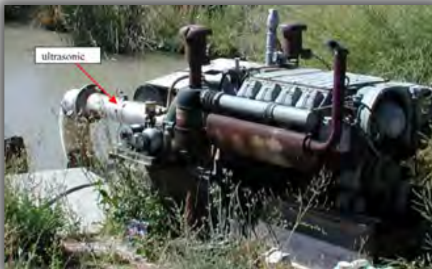
Figure 1: Bullen Farms Pump #43 (courtesy: Utah Division of Water Rights).
