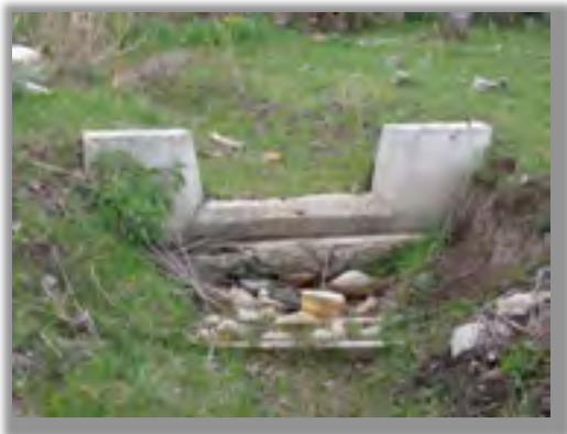
Cipoletti Weir (Clearcreek, UT)
