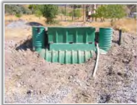
Figure 2: Textile Filter at USU Demonstration Site
