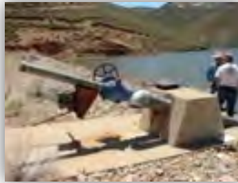
Air vent intake & gate control (Woodruff, UT)
