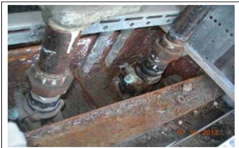
Sump Not Liquid Tight
