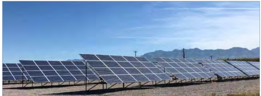
Figure 1: Community solar array installed adjacent to the Logan City Wastewater Treatment Lagoons.
