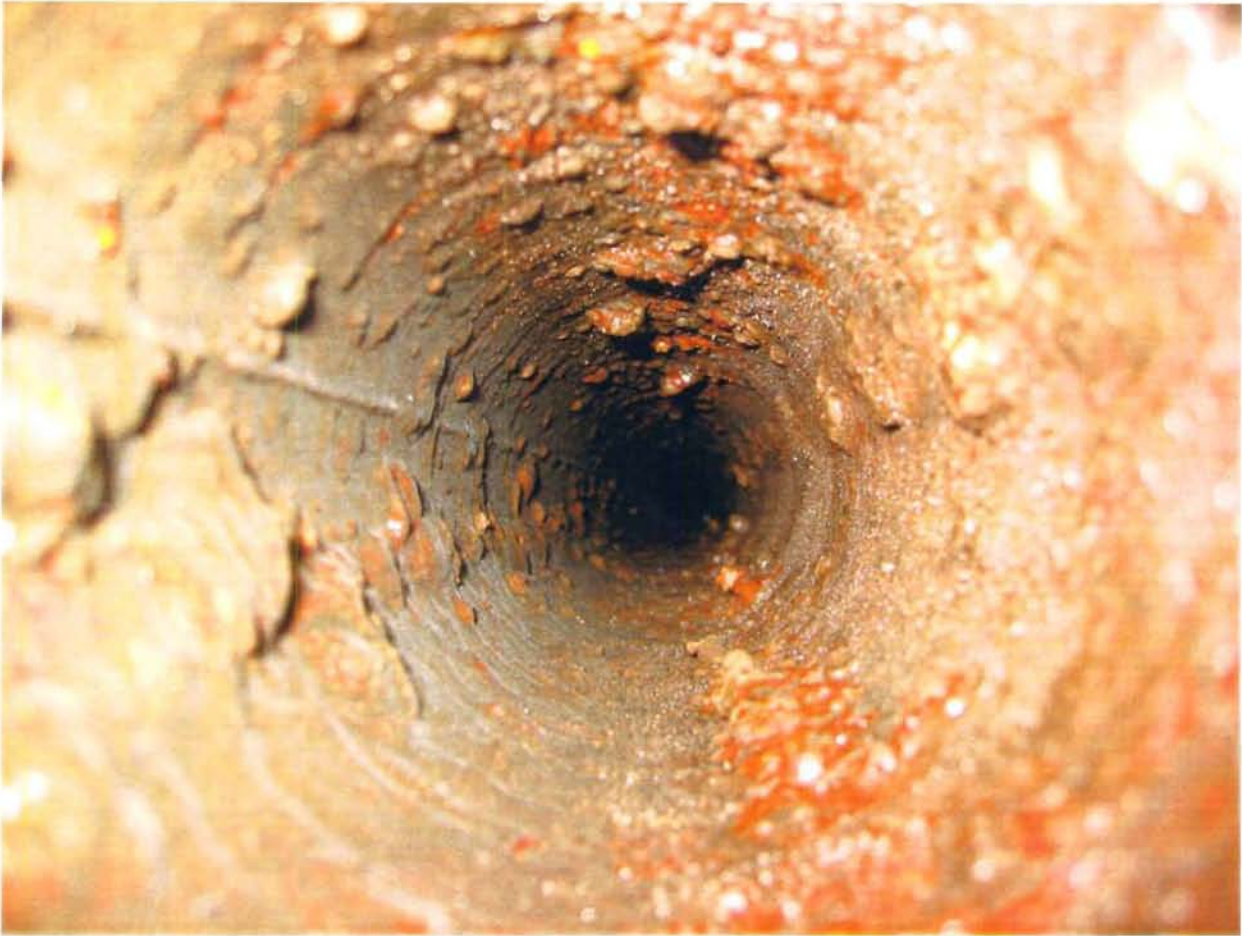
Figure 2. Four-Inch pipe picture provided by Weber Basin Water in Ogden, Utah.
