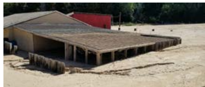
Pasture buildings and 6-foot-high fence inundated with sediment. Photo by Ben Erickson, June 7, 2018.
