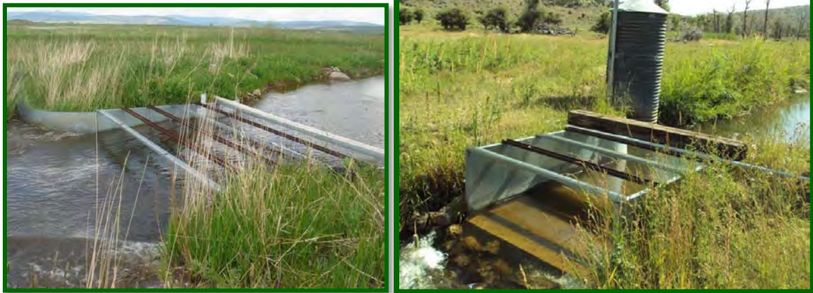
Examples of ramped flume flow measurement structures in the Upper Bear River Irrigation System.
