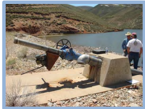
Air vent intake & gate control (Woodruff, UT).
