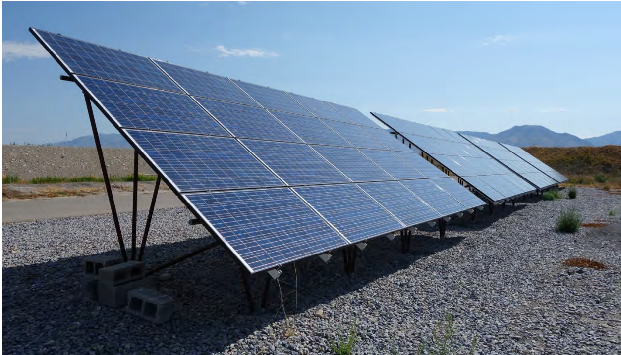
Figure 1. Solar array installed adjacent to the Logan City Wastewater Treatment Lagoons.
