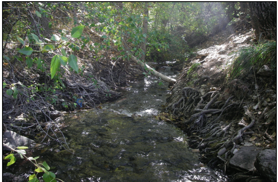
Top: Terrace erosion at outside of bend. Bottom: Low bank/root zone erosion.
