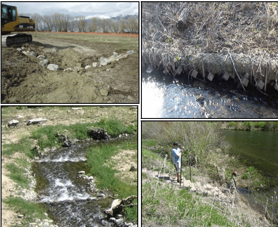
Figure 4.6. Photographs of grade-control, bank-stabilization, and access-control techniques. (Top left: construction of a vortex rock weir. Top right: A-jacks toe protection [image from Schueler and Brown 2004]. Bottom left: downstream view of two vortex rock weir structures. Bottom right: steps that provide stabilized stream access.)
