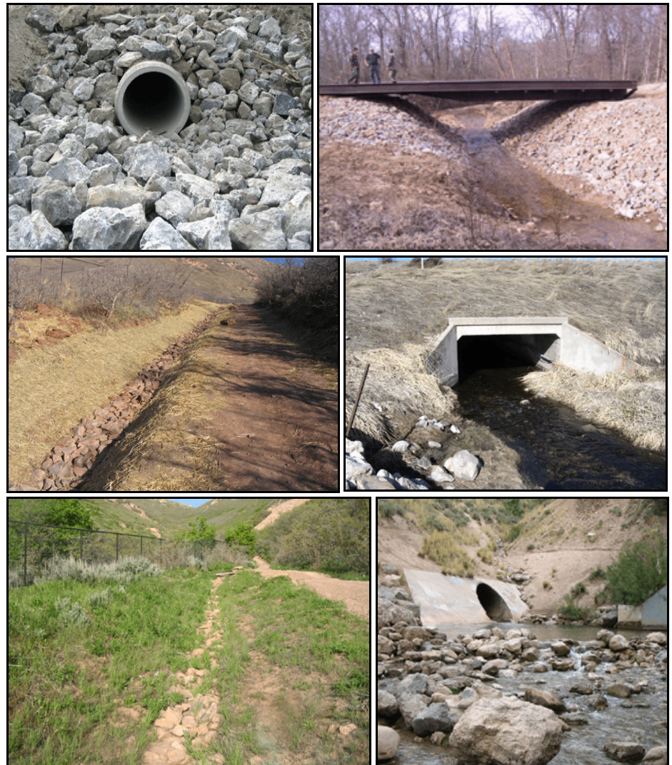
Figure 4.5. Photographs of outlet protection and stream crossing techniques. (Top left: rock outlet protection. Top right: stream crossing using a bridge made from a recycled railroad flatcar. Middle left: vegetated rock-lined swale immediately following construction. Middle right: stream crossing using an open-bottom box culvert. Bottom left: vegetated rock-lined swale in second growing season. Bottom right: tailwater pool at culvert outlet.)
