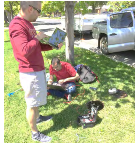
USU PhD students Camilo Bastidas and Nour Attallah install a smart water metering data logger on a residential water meter in Logan, UT
