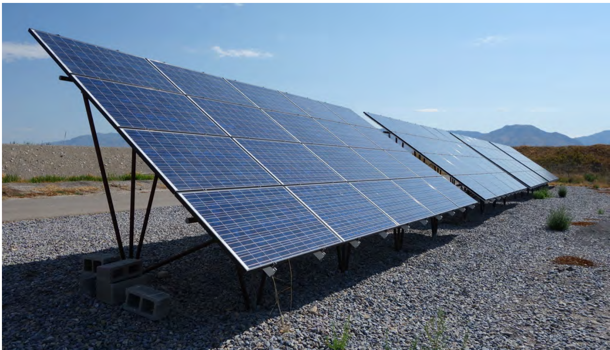
Figure 1. Solar array installed at the Logan City Wastewater Treatment Lagoons
