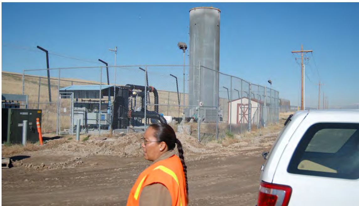
Figure 1. Flare at landfill gas recovery system at the Salt Lake Valley Solid Waste Management Facility
